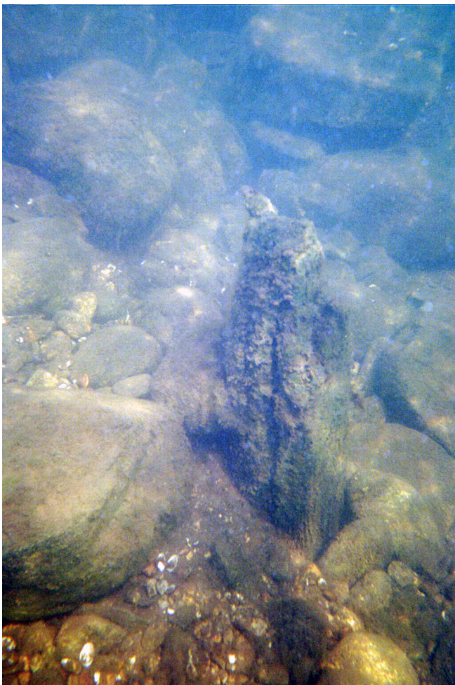
(Left Picture) One of two Wooden Pilings found at the base of the Foundation
