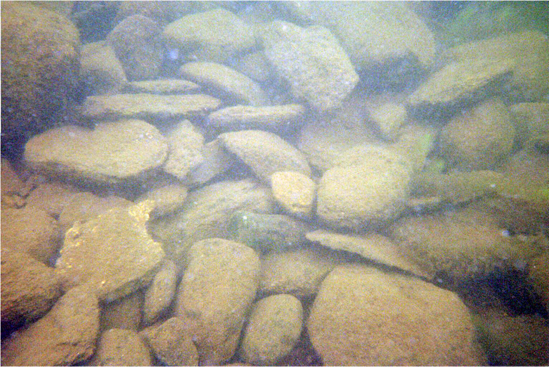
Remaining Loose Foundation
