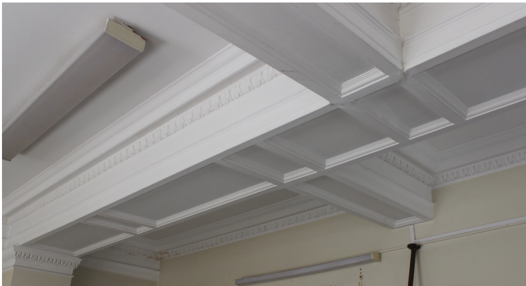
Figure 22 Detail of the downstands to the ceiling over the northern part of the southern room.
