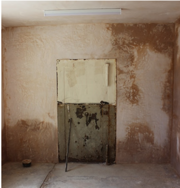
Figure 23 Former safe door within the small room to the rear of the southern room.
