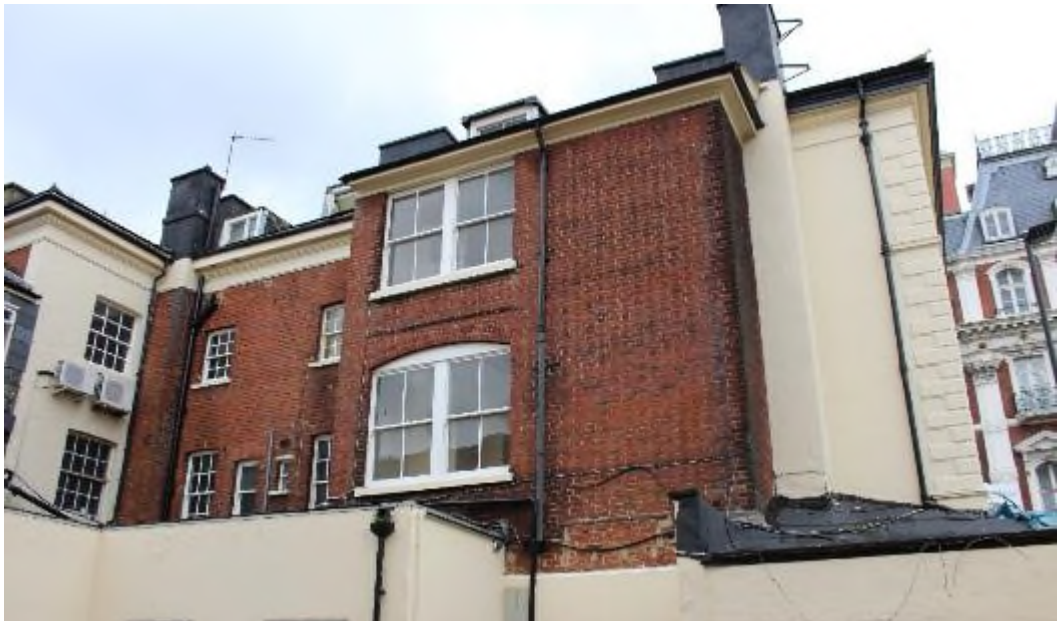
Figure 18 Rear elevation of the southern part of the Terminus Terrace range. The projecting brick element with the double sash windows is the 1907 service stair addition. The recessed brickwork to the left is the original rear elevation of the wider southern part of the building.
