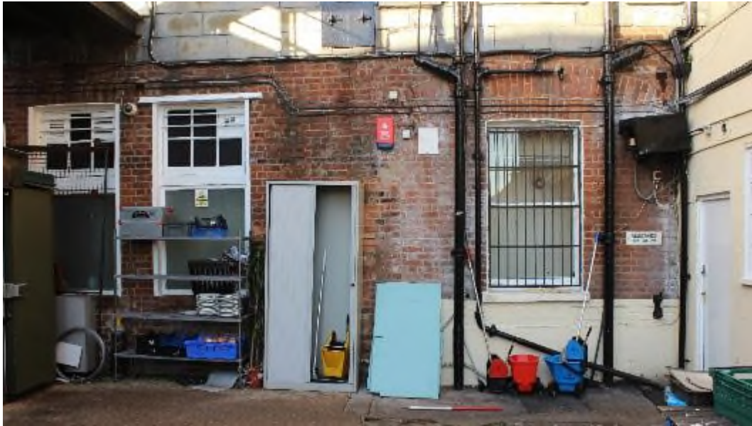
Figure 16 Rear elevation of the Oxford Street range showing the blocked carriage arch opening to the right with a two-pane sash window inserted.
