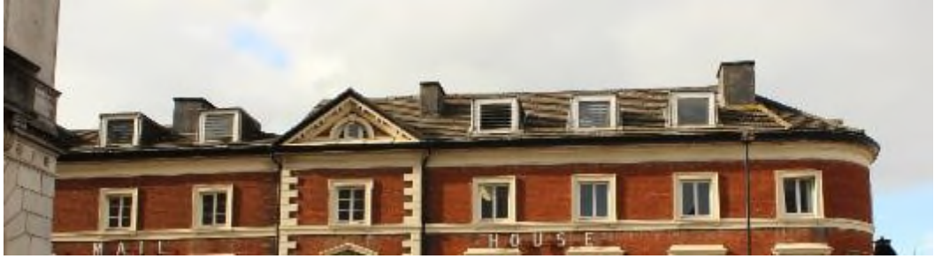
Figure 14 The roofs of the Terminus Terrace range of Royal Mail House showing the change in roof form.
