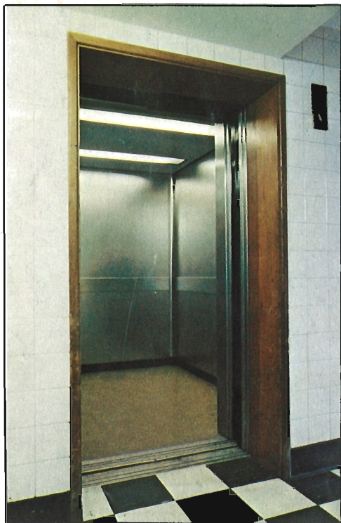
Service lift at Royal Garden Hotel
