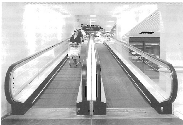
First Otis travolators in Ireland at the Merrion Centre near Dublin.
