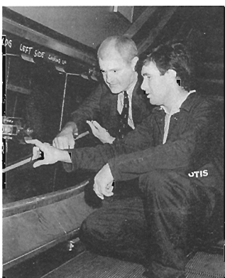
Brian King chats to charge hand Chris Hackett when he went to see modernisation work at a London underground station.
