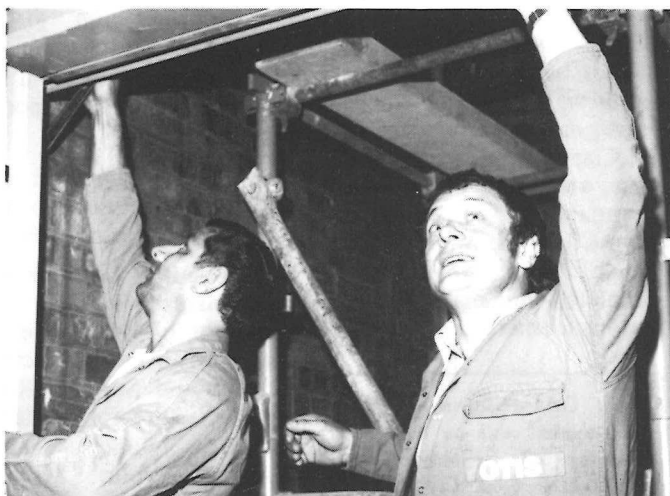
John Barns (left) senior fitter recently returned from Nigeria with mate Alex Baron. They are working in an disused hat factory which is being refurbished and converted into offices.
