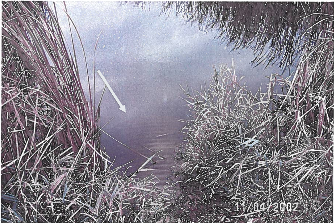
Figure 16. Obstructed culvert. This picture was taken during a period of dry weather in fall of 2002. Imagine what this looks like in the spring rainy season.
