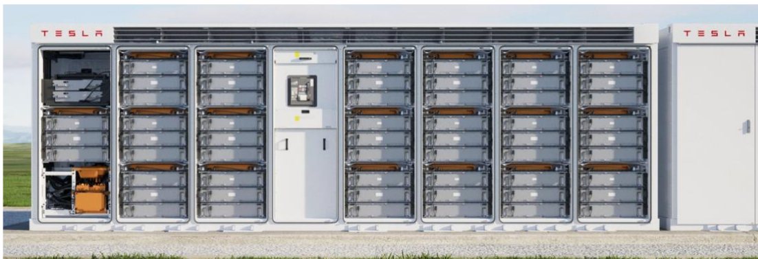
Multiple Tesla Energy Storage System Components within a Tesla ESS Container
