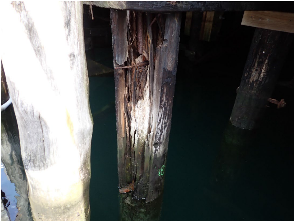
Split and rotted timber support pile.
