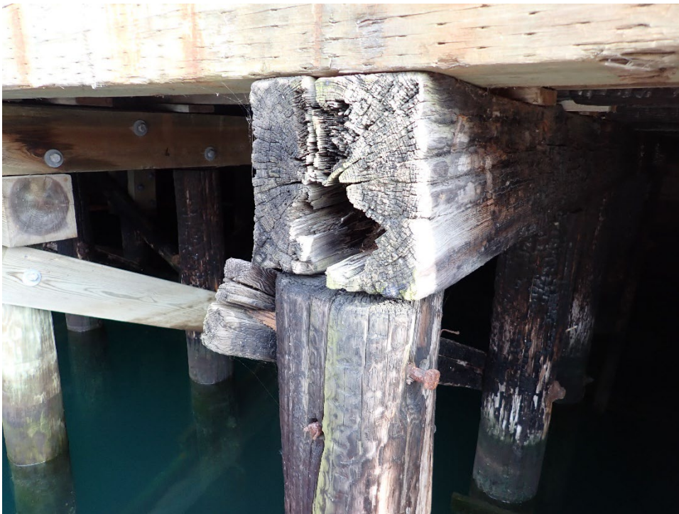
Dry rotted timber pile cap.
