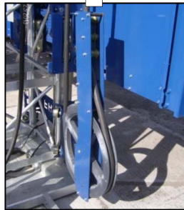
Cable guide trolley
