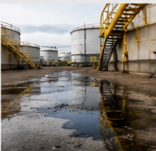
STORAGE TANK LEAKS
