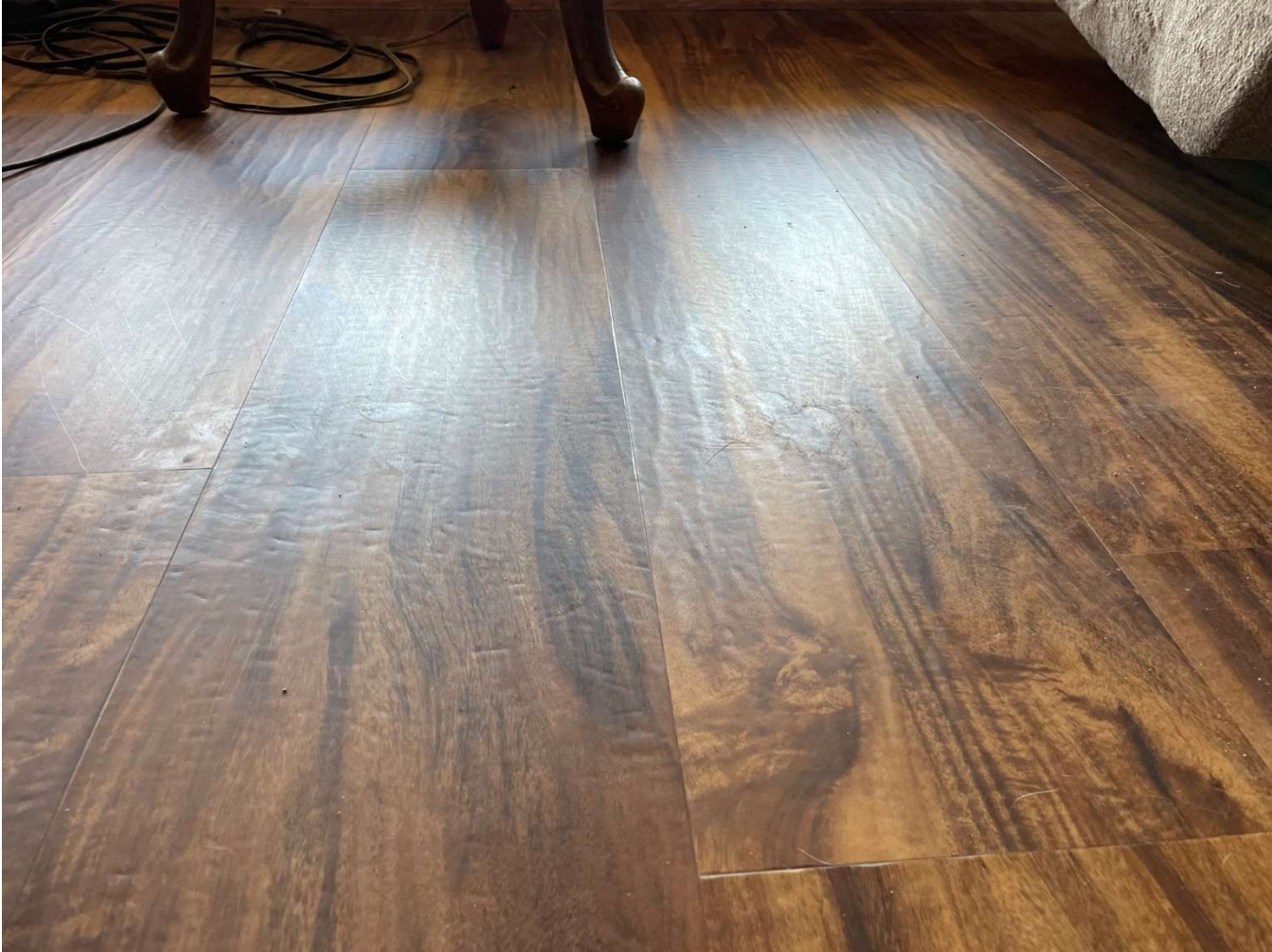
Scuff marks before cleaning
