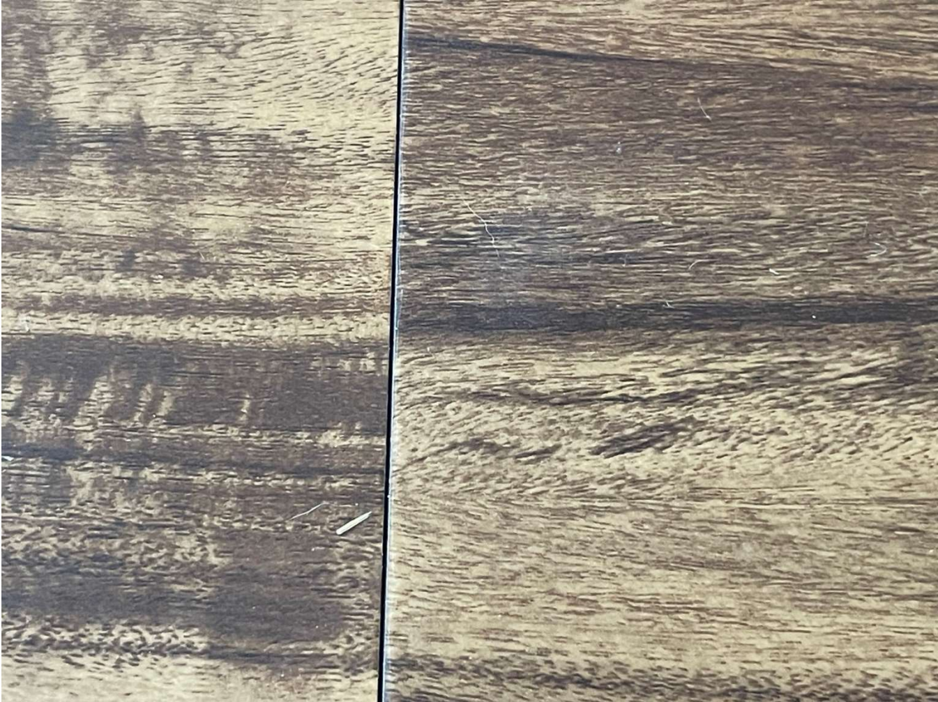
Gap at end joint
