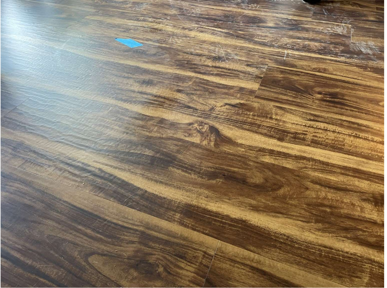
Larger cleaned area- haze still present
