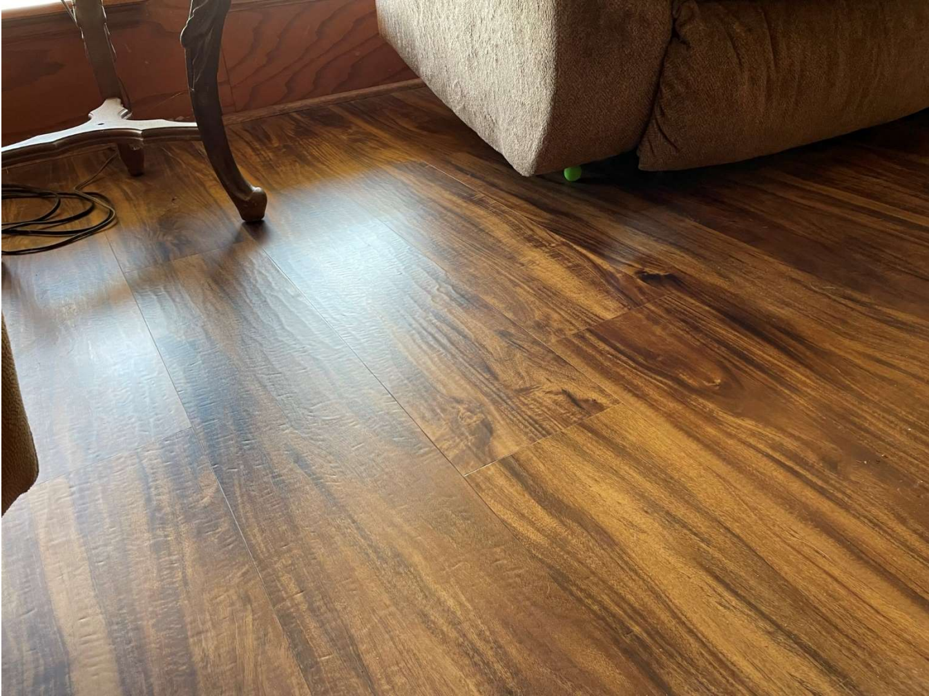
Scuff marks after cleaning
