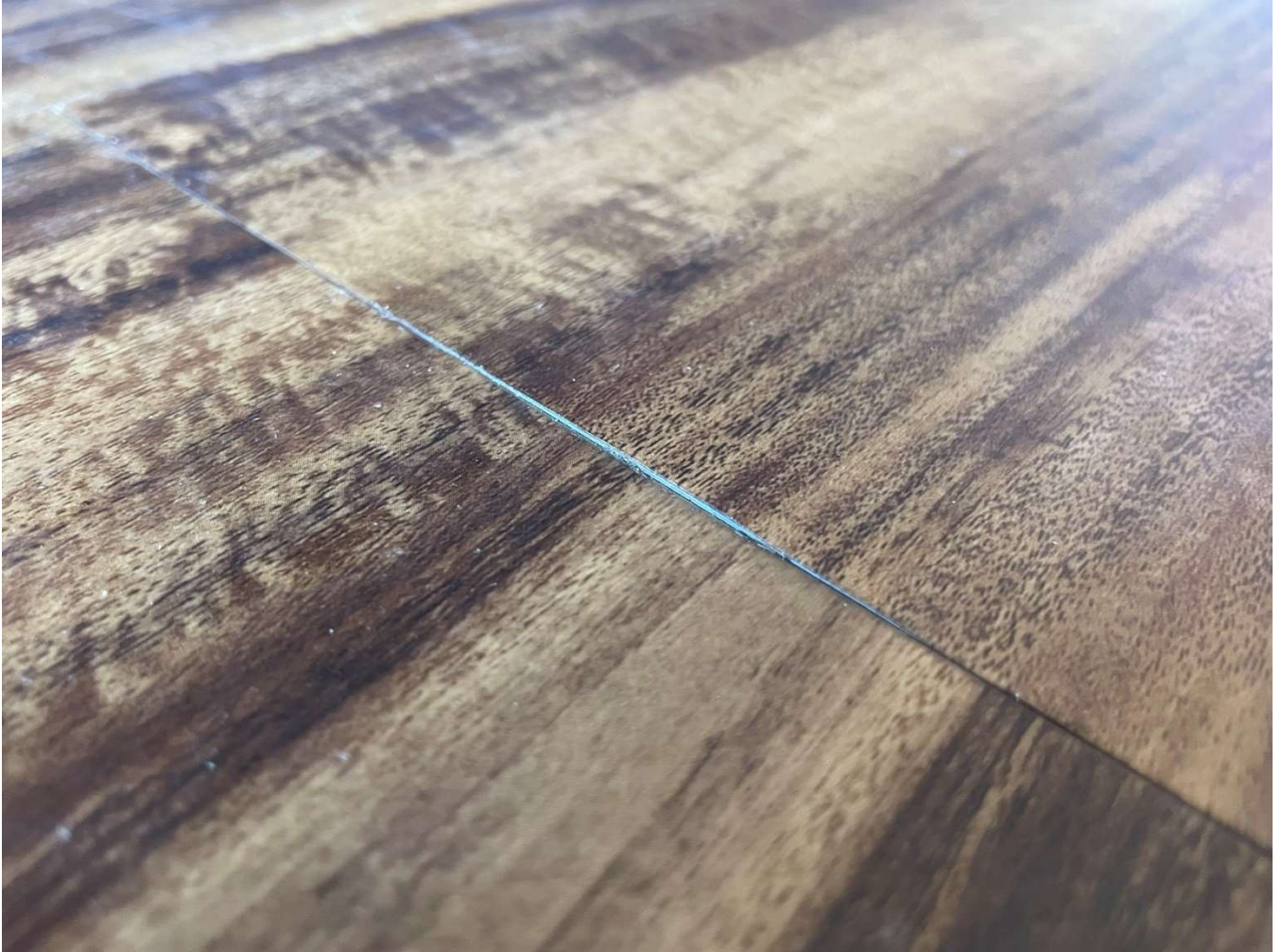
Disengaged end joint- deflection at joint
