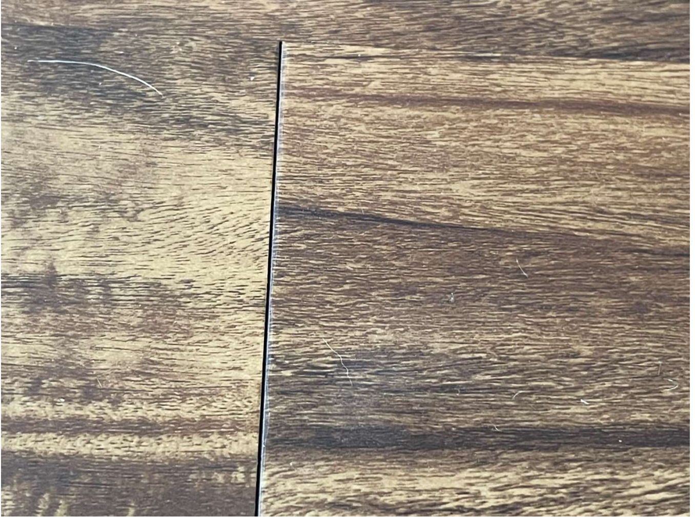
Gap at end joint
