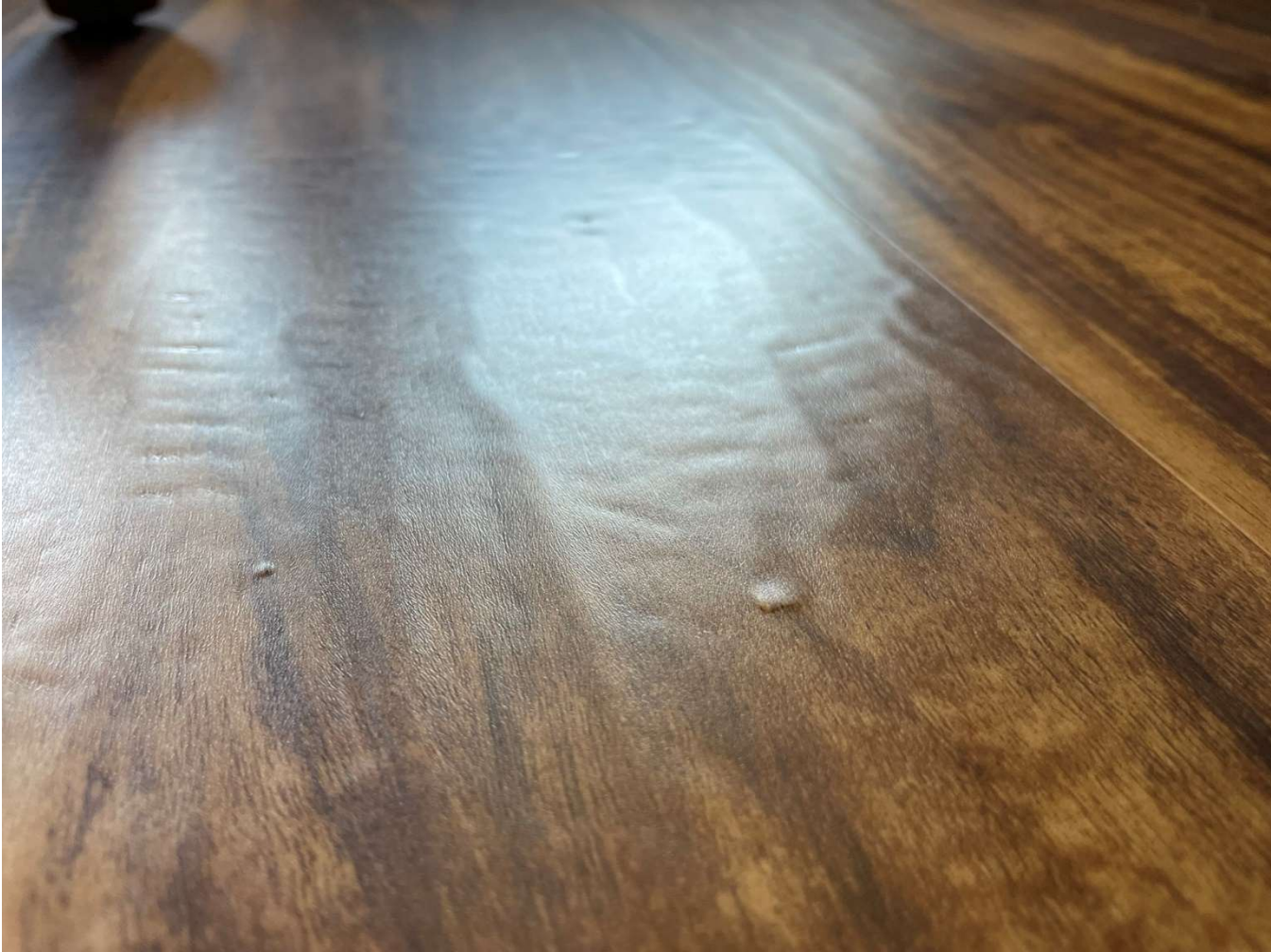
Telegraphing spots- possibly from debris trapped beneath flooring
