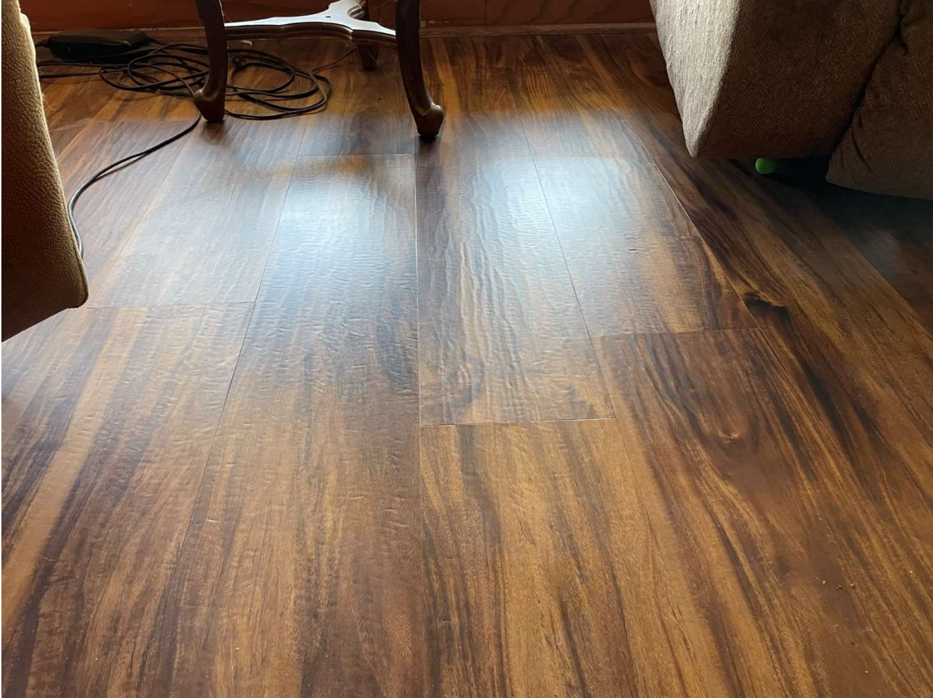
Scuff marks after cleaning
