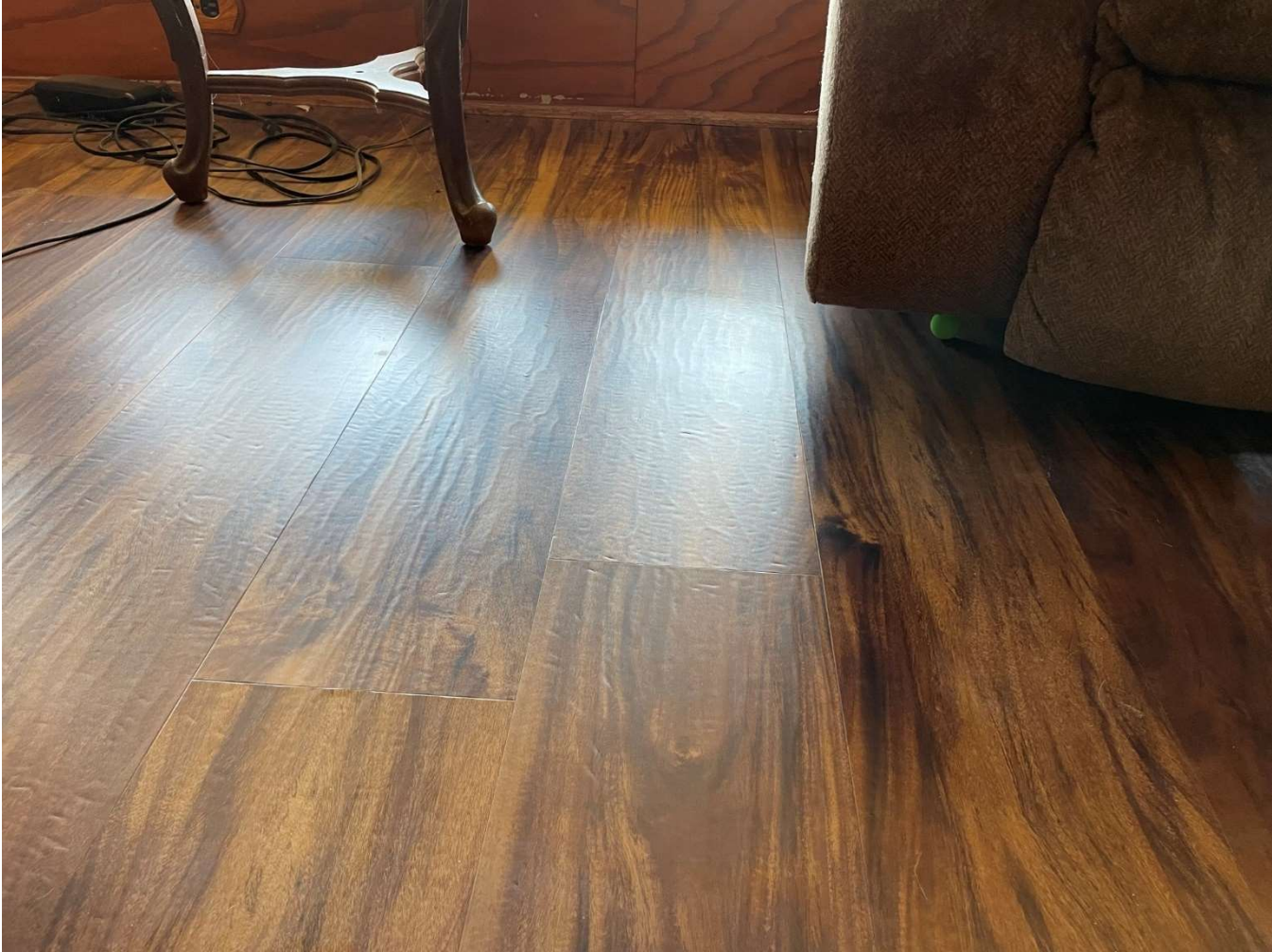
Scuff marks after cleaning
