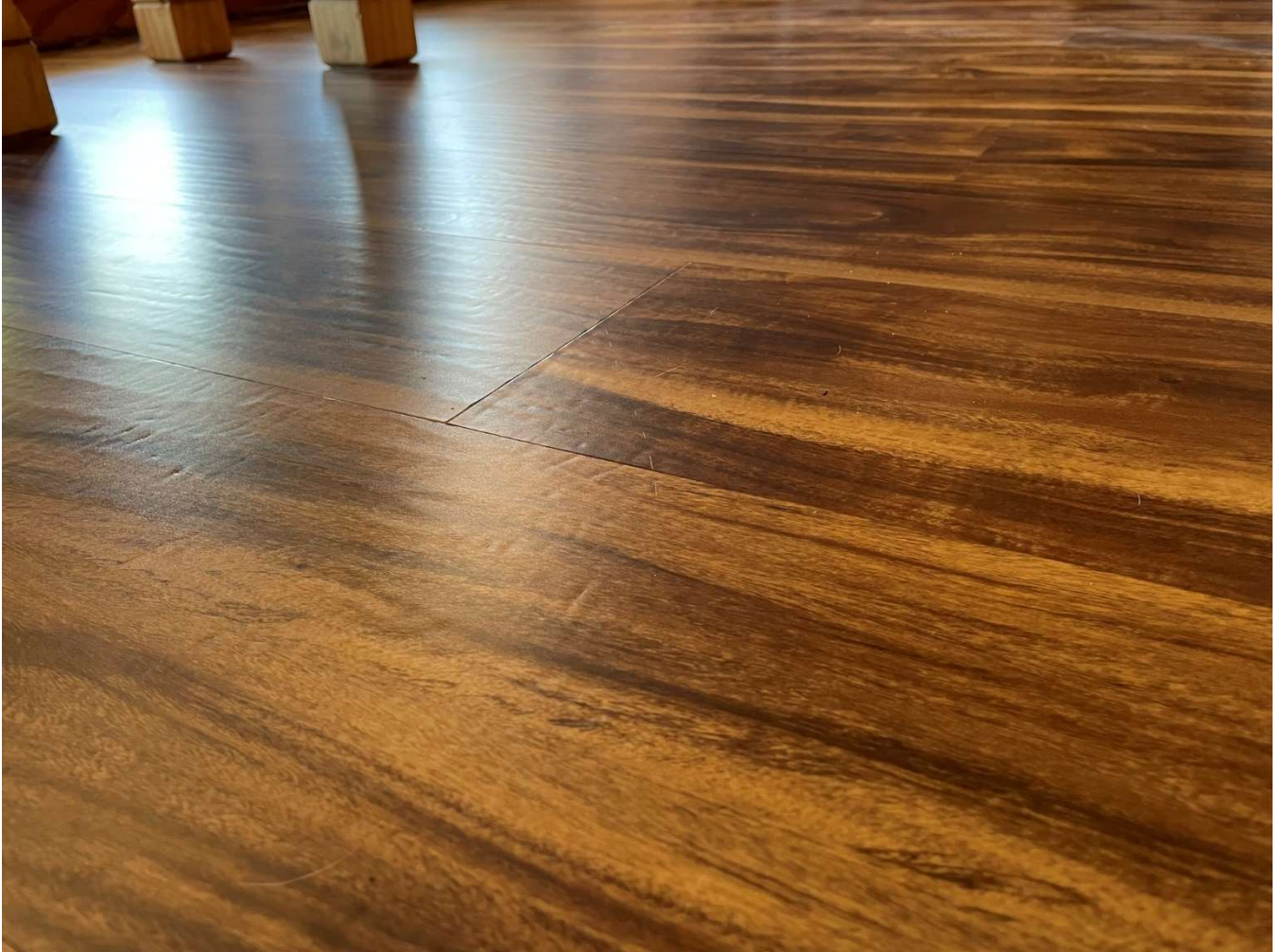
Ramp at end joint- broken locking mechanism
