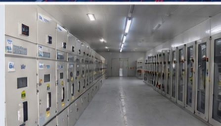
LCC – Outdoor Substation (Internal)
