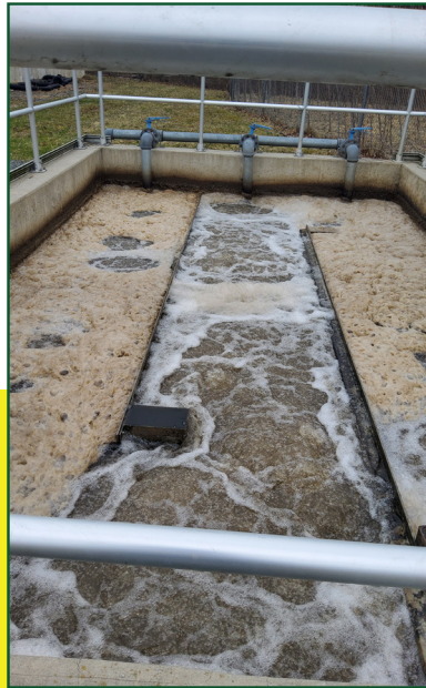
The same tank, filled with dirt, before the expensive cleaning work that the village had to put in.
