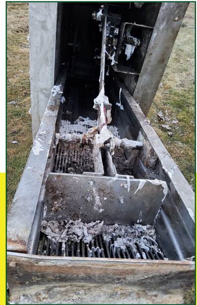
Over $200,000 (!) in machinery was changed this year because of the use of so-called "flushable" wipes!
