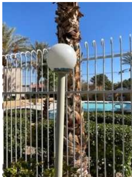
Replacement of the Light Fixtures has been included in the Study. The estimated useful life is approximately 20 years.
