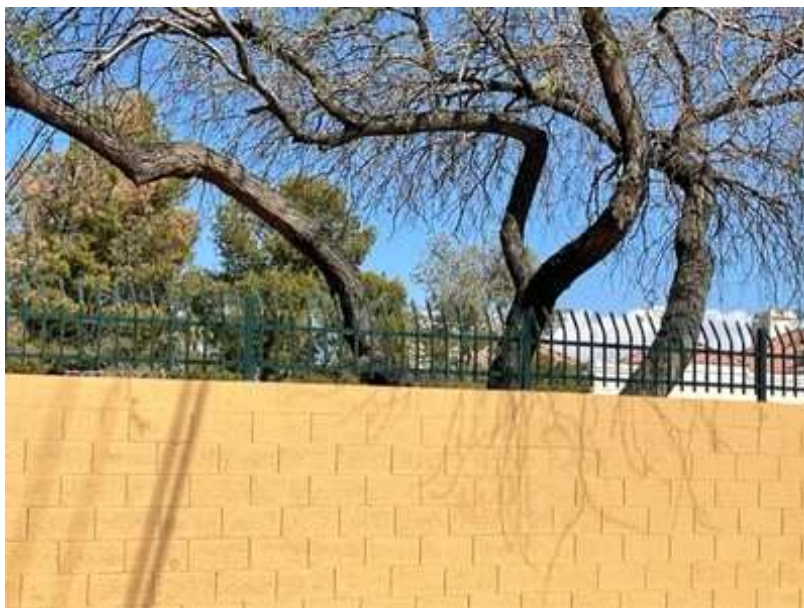
The Perimeter Wall and Landscaping are maintained by the Homeowners Association. Perimeter Wall Repairs have been included in the Study as an allowance, to be done as needed.
