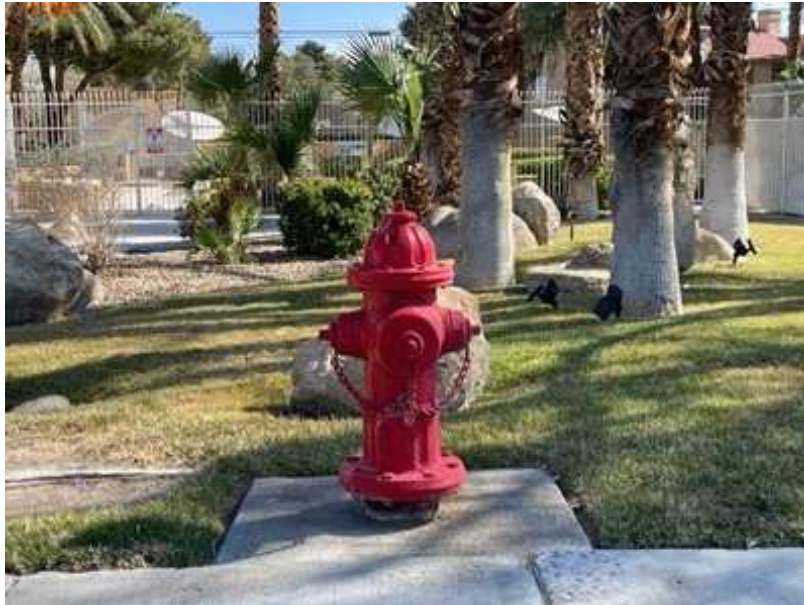
Fire Hydrants are maintained by the Association. Replacement has been included in the Reserve Study.
