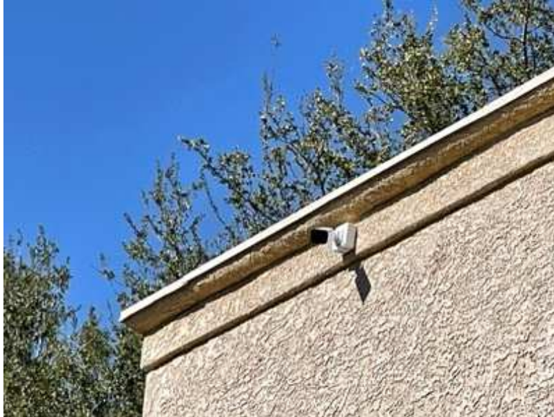
Security Camera Repairs or Replacement has been included in the Reserve Study to be done as needed.
