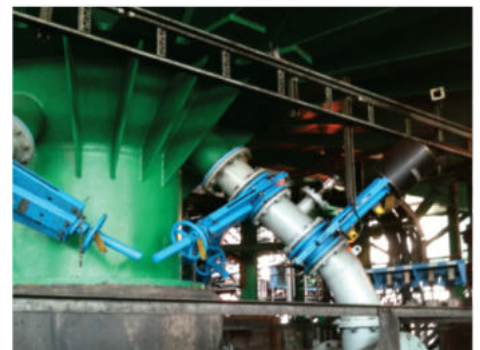
Coal Washing Plant
