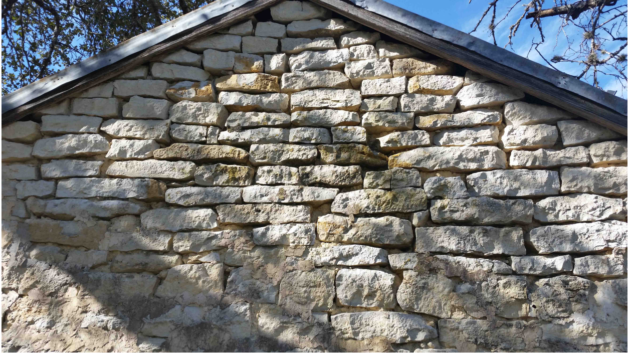
Mortar Damage: Rear of Building
