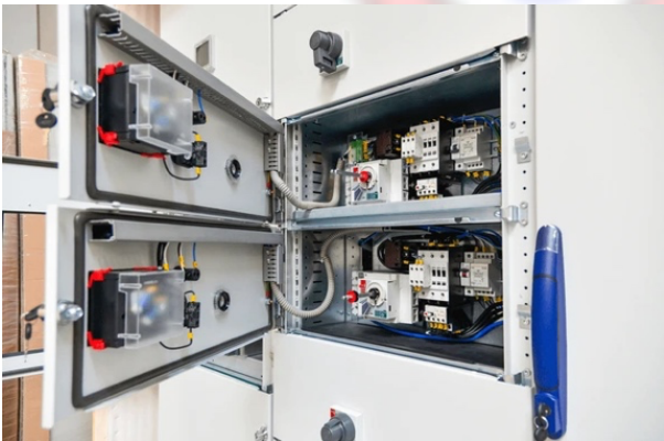
Figure 1: Protection & Control Relays
