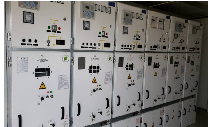
Figure 2: LV Panels & Components
