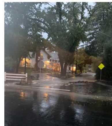
Water overflowing the culvert over the road at El Centro and Avenida Nueva
