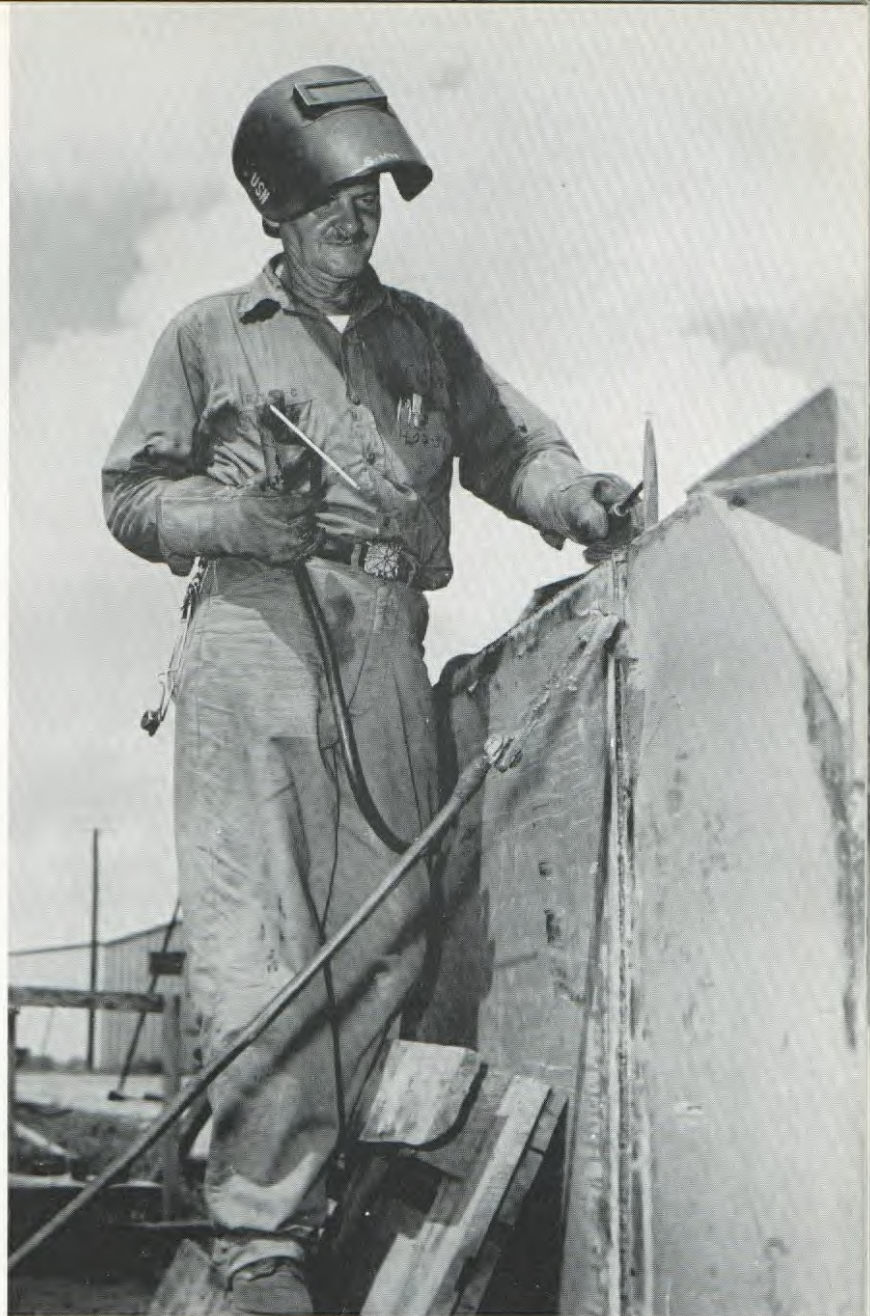
SEABEE welder, one of 114 enlisted men in the Mobile Construction Battalion (Special), practices assembling art.
