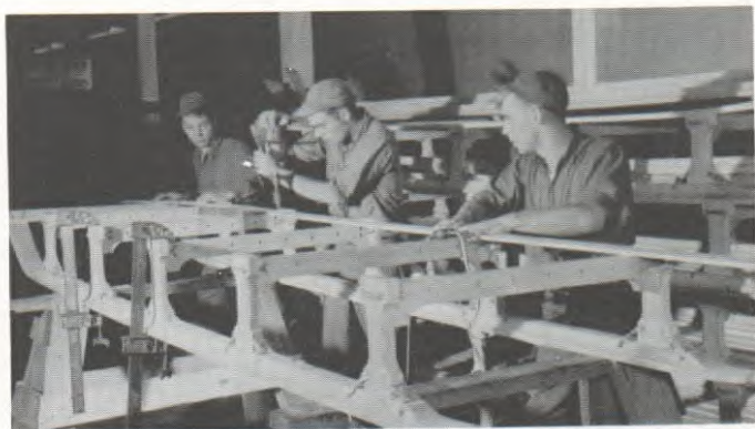
"CAN DO" pays off as Seabees Jack Steward, BU3, Robert Norwood, BU2, and Richard Prescott, BU3, construct one of ten dog sleds to be used at Pole for rescue, reconnaissance.
