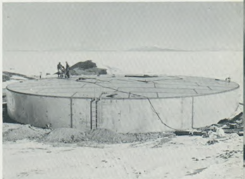
fuel transfer lie on icy incline. Upper right, finished tank to hold 250,000 gallons received from the NESPELEN.
