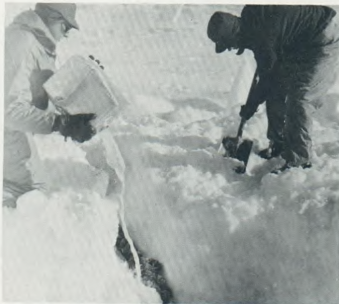
BURIAL under layers of snow secures deadman; water poured over ropes and log freezes rock-hard in five hours.
