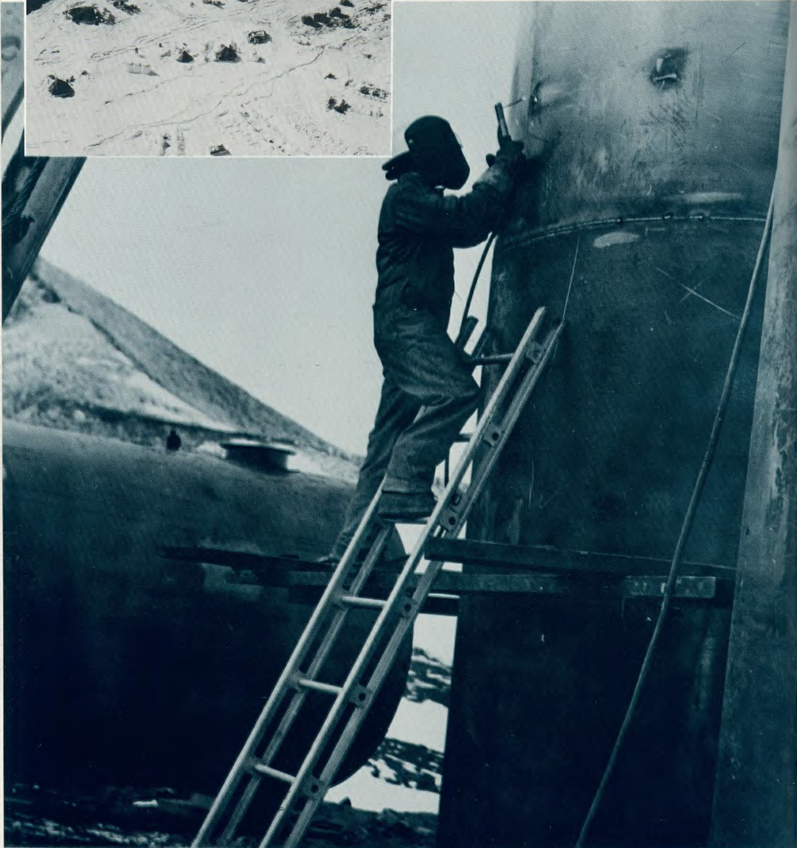
HUT POINT HAD FUEL FARM SYSTEM, TOO. CHICAGO BRIDGE & IRON WORKS WELDER SEAMS TANK
