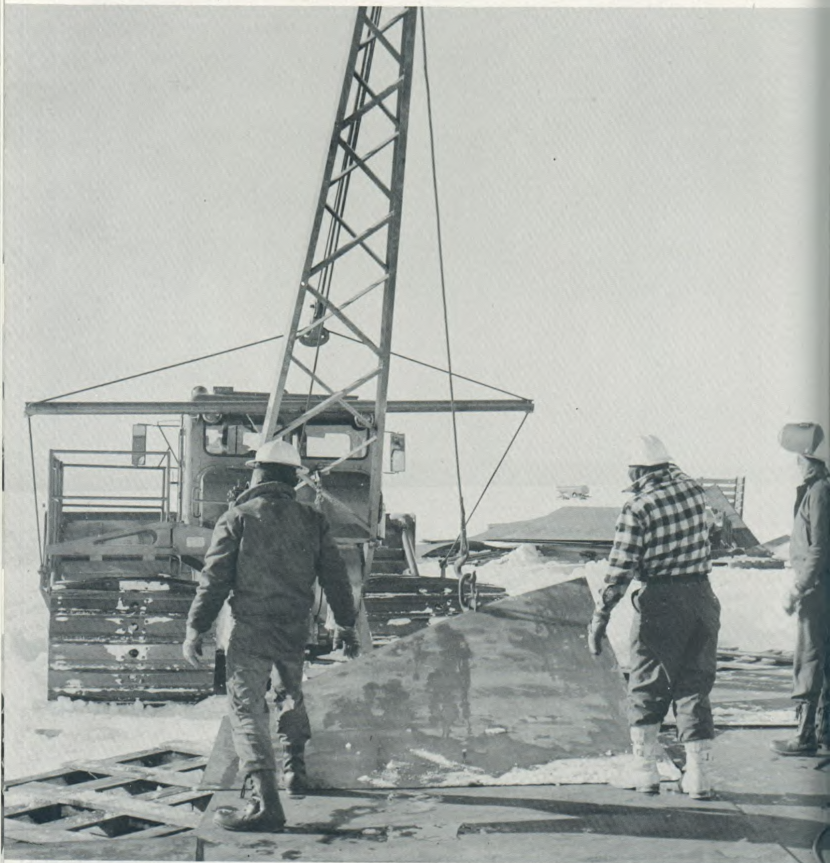
FLOOR PLATES of 250,000-gallon fuel tank being erected at Little America V are lowered into place by crane.
