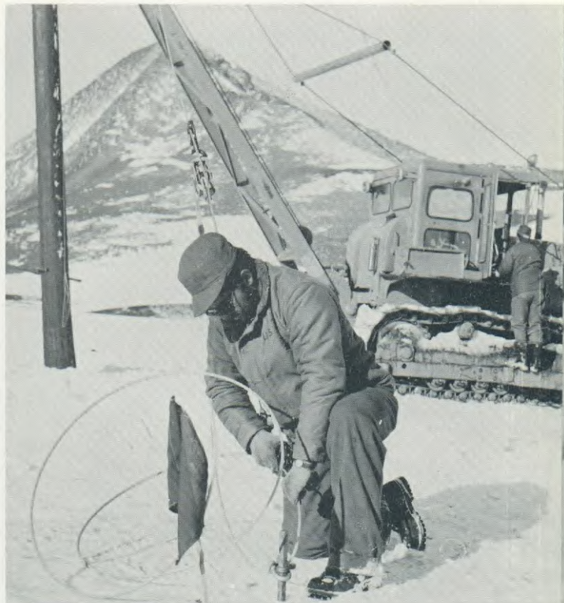
in service. Upper right, construction men installing electric power lines with D-8 tractor to help raise pole.
