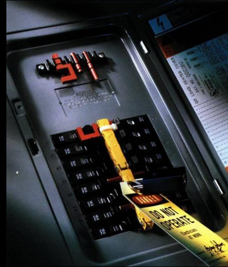
Locked out circuit breaker
