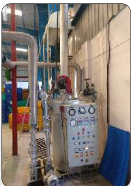
HOT WATER / PT PIPING
