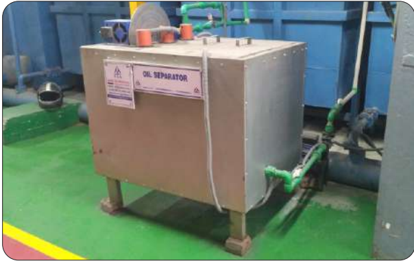
OIL SEPARATION SYSTEM
