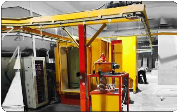
CHAIN CONVEYORISED POWDER BOOTH
