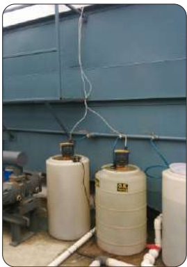
AUTO DOSING SYSTEM
