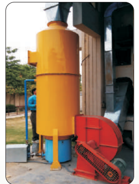
FUME EXTRACTION SYSTEM
