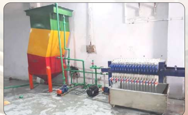
SLUDGE SEPARATION SYSTEM
