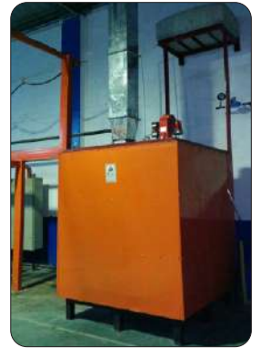
HOT WATER GENERATOR
