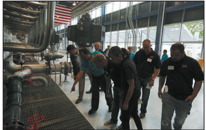
Water plant Senior Technician Jose Ronquillo (second from left) shows feed water piping that feeds the reverse osmosis booster pumps at the KBH Desalination Plant.
