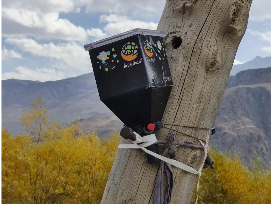
Katidhan light installed at Holiyal
