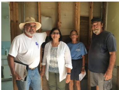
John Rickards (on left) from Alabama's Habitat for Humanity helped with repairs.
