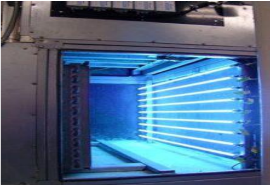
UV-C Germicidal Lighting Added to Commercial Air Handler
