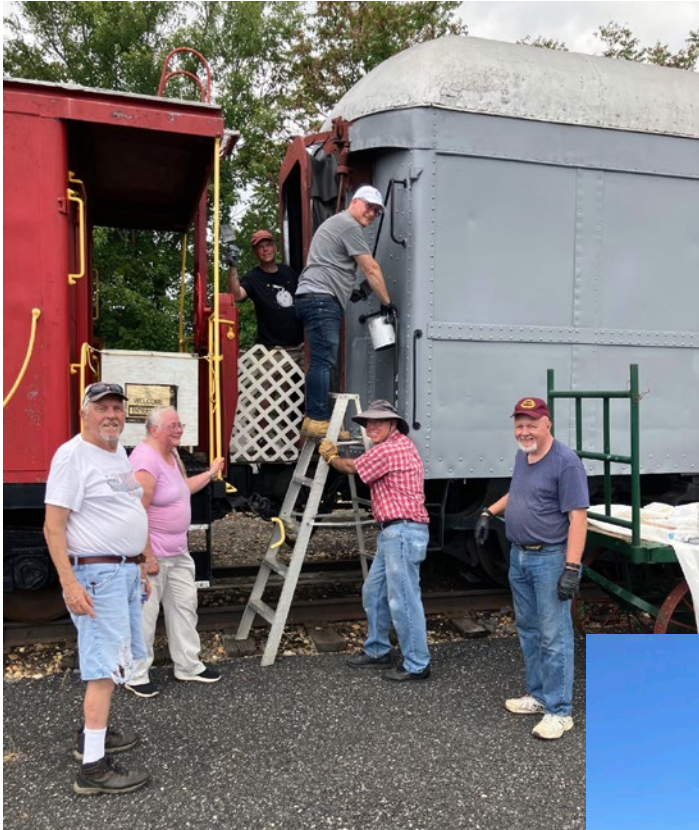
Left: The Paint Crew. Below: The Paint Crew applying Tucson to B-60 on Sunday afternoon.
