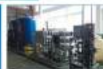
Reverse Osmosis Water Treatment
