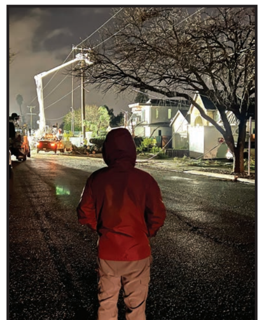
Local residents patiently look on as PG&E attempts to restore power in the Morgan Park neighborhood.
