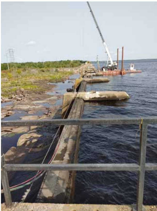
Spillway Restoration: We specialize in the meticulous restoration of spillways. Our expert team handles projects like this 550 feet across, 30 feet tall, with up to 8 inches thickness of dry-mix shotcrete. All work was efficiently carried out using crane and barge equipment.
