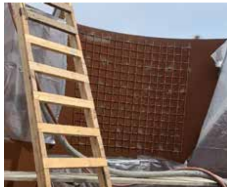
ABOVE: Rondout Bypass Tunnel | New York, NY. LEFT: Shotcrete as Roadside Slope Protection in Brazil | SP 333 Highway, São Paulo, Brazil
