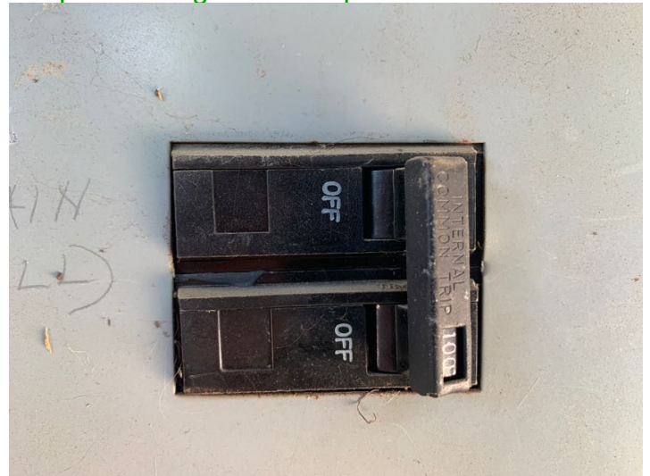
Main electric disconnect was rated at 100 amps
