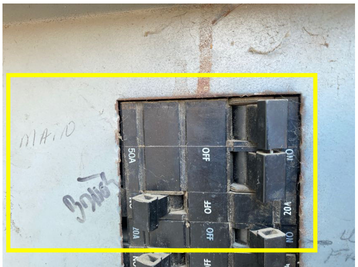
50 amp breaker installed
