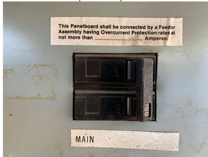
Main service disconnect was rated at 100 amps
