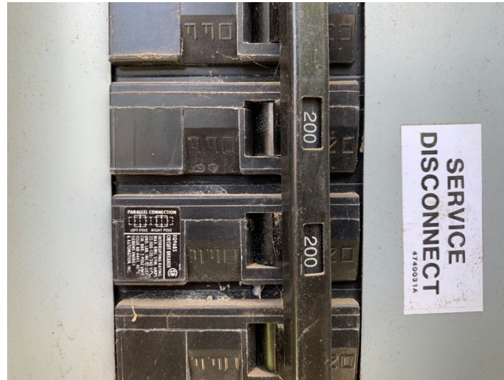
Main service disconnect is ready to 200 amps
