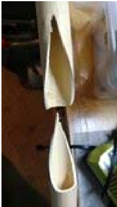
One of two broken pipes
