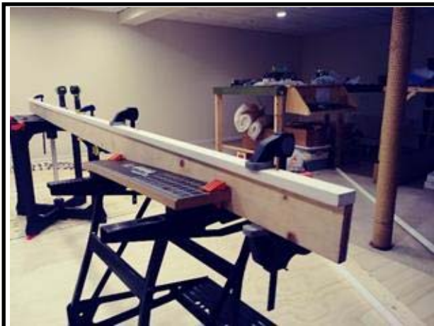
L-girder under construction. Using 1" x 4" lumber and 1" x 2" flange giving it remarkable strength
