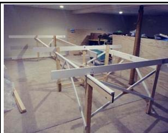
L-girders being attached to the leg assemblies using deck screws and 1/4" bolts. Notice the "1 x 2" bracings
