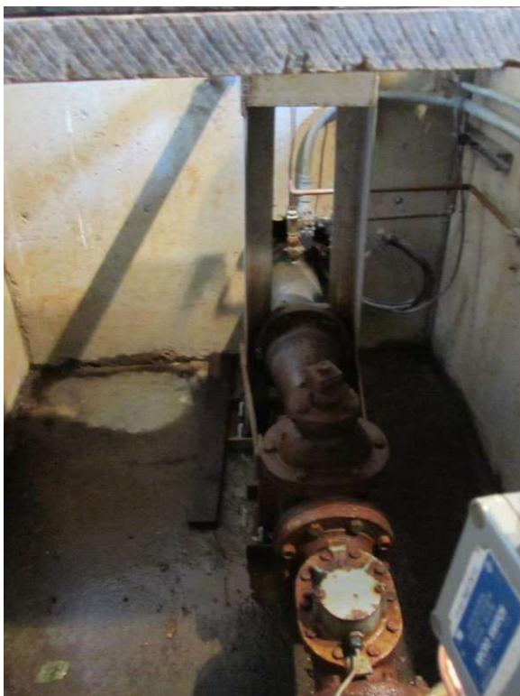
Well discharge piping.
