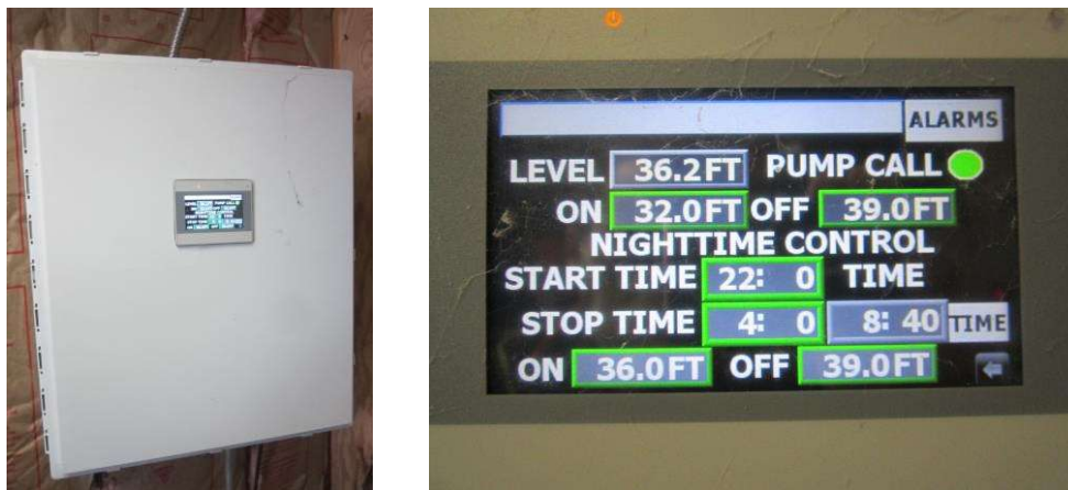
Reservoir level and well pump control panel and interface screen, in the High Zone pump station.
