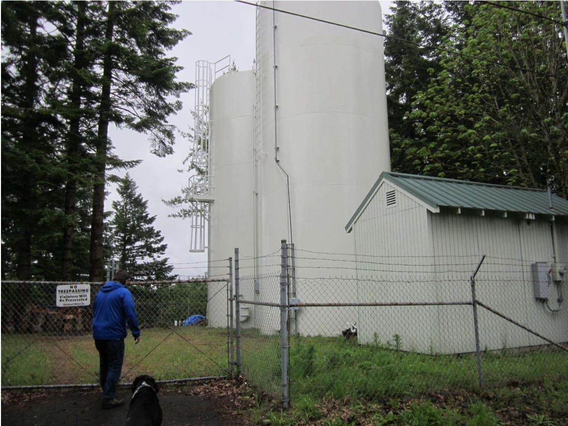
General reservoir and pump station site area as viewed from SE Castle Court.
