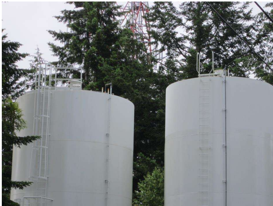
Reservoir exterior upper areas as viewed from SE Castle Court, Reservoir 1 on right and 2 on left.
