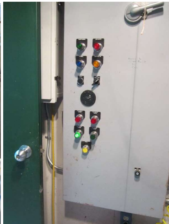
Well pump status lights and HOA switch.
