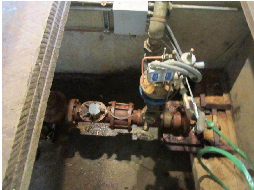
Well discharge piping and solenoid-operated pump control valve.
