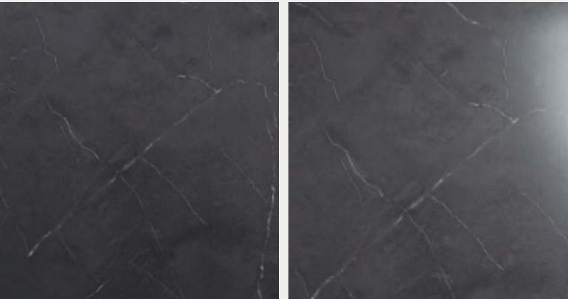
A117 Cement Cracks
