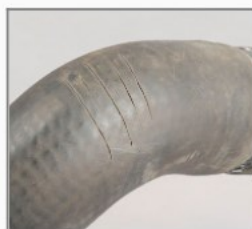
Ozone Damaged Hose
