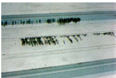
Figure 1. Black storage stain on a GALVALUME ® roof panel.
