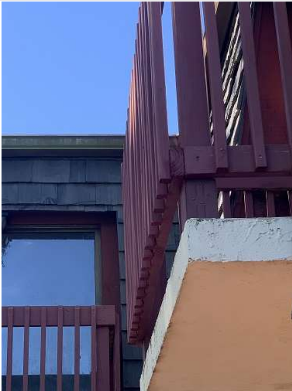
Balcony: posts attached at the top of the stucco balcony slab
