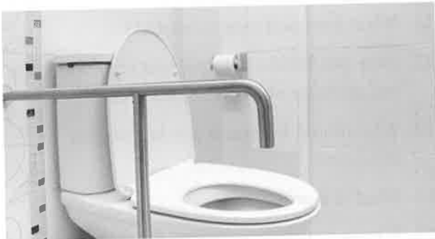
Fig. 13-44. Handrails can be installed next to toilets to promote safety. The HHA should report if these assistive devices are needed.
