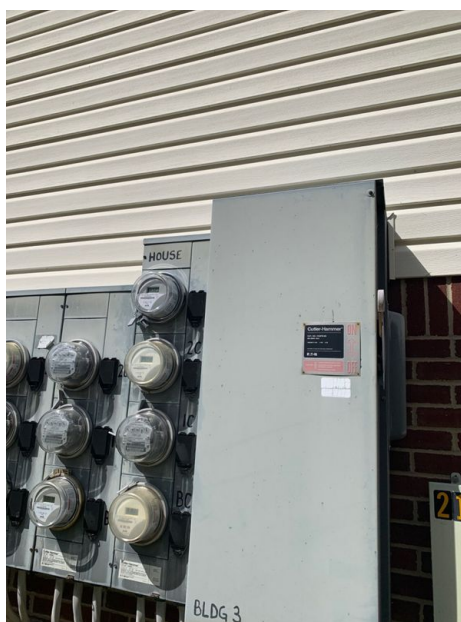
Service Entrance Conductors: Electrical - Main Shut off
