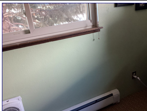
The bottom of the windows in the Bedroom were 44" or more above the floor level. This restricts egress in case of an emergency. This is a safety concern. I recommend consultation with a qualified contractor to address the issue.
