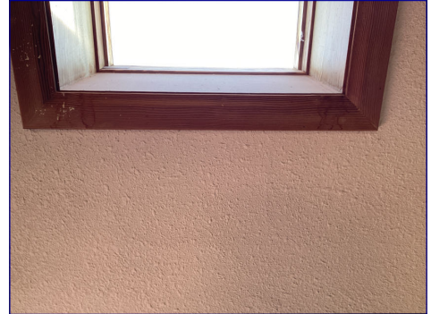
There were indications of moisture around the skylights. I recommend a licensed contractor evaluate and repair.
