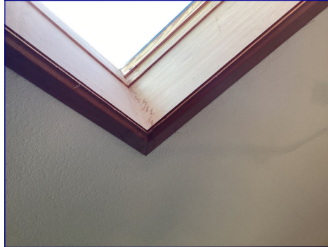
There were indications of moisture around the skylights. I recommend a licensed contractor evaluate and repair.
