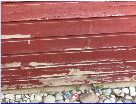
The siding needs routine repair and painting maintenance. I recommend a licensed contractor repair and paint the siding.
