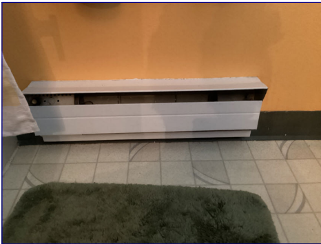
Electric baseboard radiant heat in downstairs bathroom
