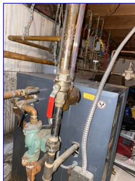
I observed corrosion on multiple parts of the boiler. The boiler worked fine. The boiler is past the normal operating life span. I recommend budgeting for a new boiler.
