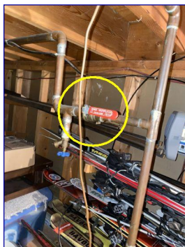
This valve is for the irrigation system.
