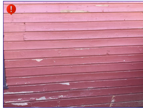
A large portion of the siding on the home is in good condition. There are places where the siding paint is peeling. The peeling paint can hold moisture and pests which can further deteriorate the wood siding. I recommend having a painting contractor evaluate the siding and repair and paint the areas that are showing bare wood and peeling paint.
