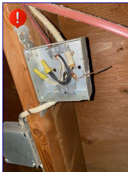
There were open junction boxes in the crawl space. I recommend having covers installed. This is considered a safety hazard.
