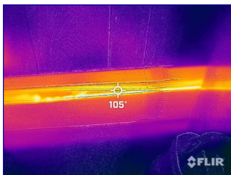
The boiler pumps hot water thru the system.
