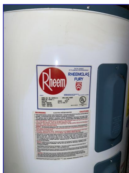
The Water Heater Data Tag
