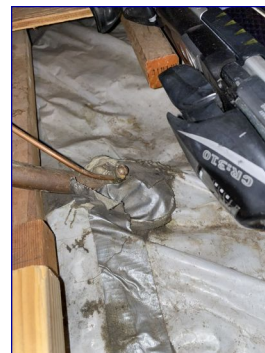
Ground wire attached to copper water pipe.
