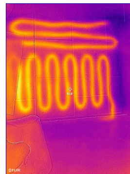
Radiant heat in the upstairs bathroom.
