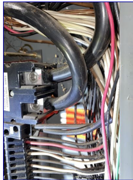
Aluminum Service Conductors
