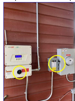
The solar system located on the exterior east wall. Emergency disconnects are in this location.
