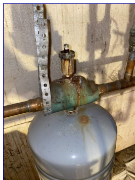
I observed corrosion on the air scoop and air vent. This could affect the operation of the expansion tank . I recommend evaluation by a licensed HVAC technician.
