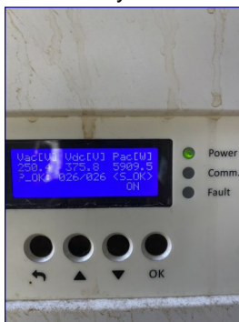
The solar system is not included in the Standards of Practice for a home inspection. Any information on the system is shared as a courtesy. The solar system appears to be operating correctly.
