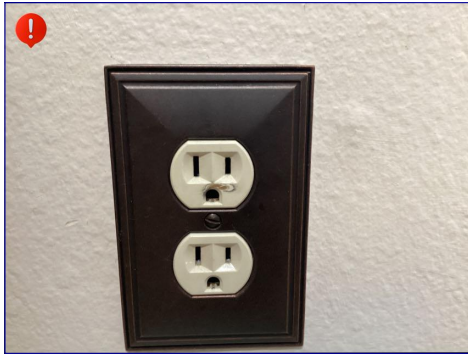
I observed a scorched receptacle. This could be a safety hazard. I recommend evaluation by a licensed electrician.
