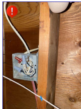
This is a second junction box without cover. I recommend installing a cover. This is considered a safety hazard.
