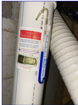
The Radon System. Installed 1998. CDPHE recommends testing for radon levels in the home every few years.
