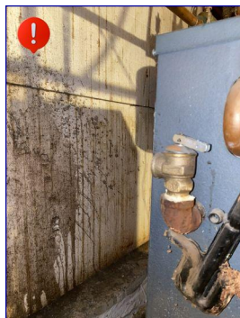
The temperature pressure release valve did not have the proper extension on it. I recommend having the proper extension added.
