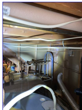
I observed wiring not attached properly. I recommend evaluation and correction by a licensed electrician for safety.
