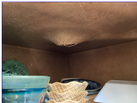
Pretty severe water damage in the top of one of the kitchen cabinets.
