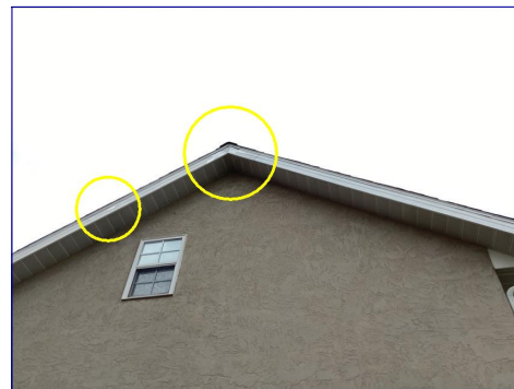
The fascia needs routine painting maintenance.
