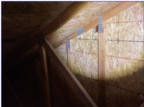
This is a hole in the wall sheathing in the attic. There is no hole on the exterior siding in this area.
