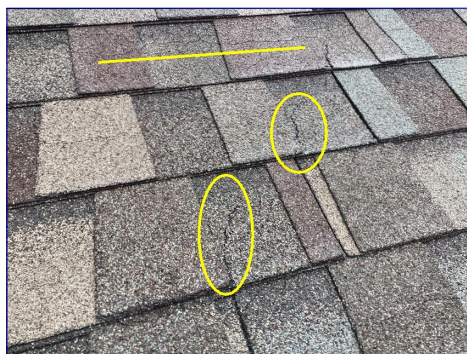
Roof covering showed signs of curling, cracking, and aging. I recommend evaluation by a qualified roofing contractor to determine the life expectancy of the roof.
