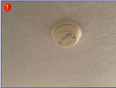
The smoke detector could be original with the house. The yellow color indicates aging of the smoke detector. I recommend installing new smoke detectors.
