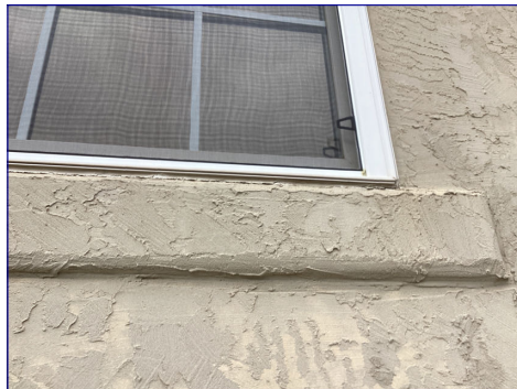
The caulking around the windows needs maintenance.
