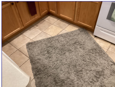
The area rug in the kitchen was taped to the floor. This limited my inspection of the floor tiles.
