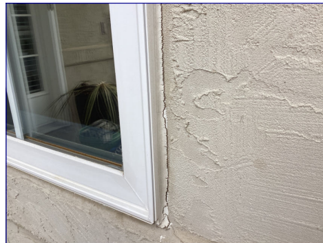
The caulking is dried and cracked. I recommend a qualified professional remove and replace the caulking. This should help protect the house from further damage.
