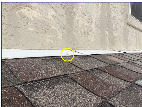
Nail pop in flashing above garage door. I recommend repair to prevent water intrusion.
