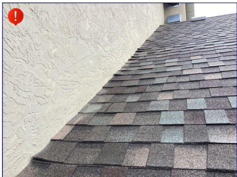
Flashing is not visible between the roof and the wall. I recommend consulting with a qualified roofer to address this concern.
