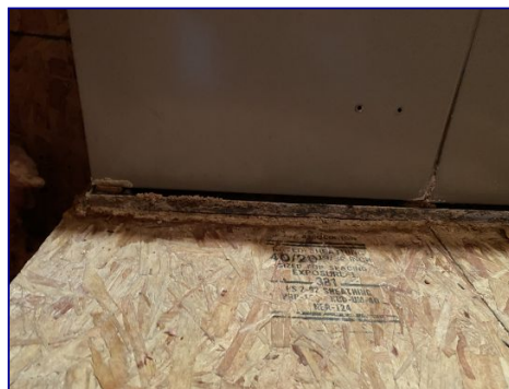
The cooling system was not tested. I tried to test the blower and nothing happened when I flipped the switch. I believe the disconnected water line in the bathroom runs to the evaporative system. I recommend a licensed HVAC technician evaluate the system to ensure it works properly.
