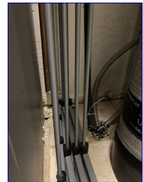
TPR Valve is piped to the floor correctly
