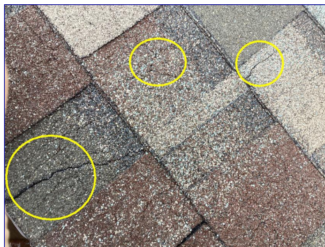
The shingles are showing signs of age through cracking. I recommend consulting with a professional roofer to determine the life expectancy of the roof.
