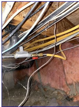
This is another Gas shut off valve. This one is located in the crawl space.
