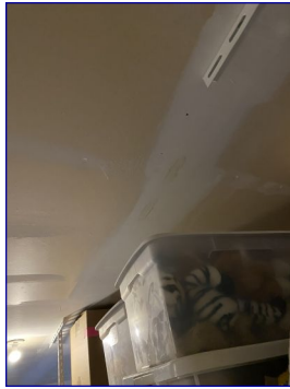
Additional picture of the garage ceiling water staining.
