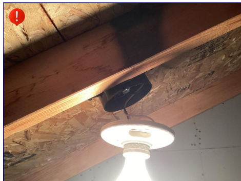
The light fixture needs to be secured to the housing.
