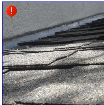
In this picture, not 757Pine Ct, the flashing can be seen between the stucco and roof. I recommend a licensed roofer evaluate the current roof, including the intersections with the walls and the flashing.
