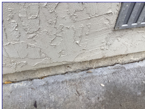
There is a gap between the patio and the house. I recommend sealing the gap between the patio and the house to help prevent water penetration.
