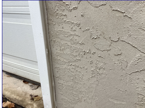
The exterior trim is in need of normal caulking maintenance.
