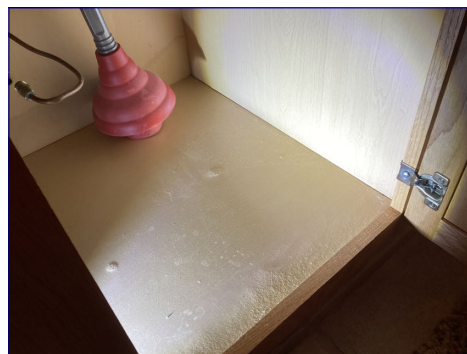
Additional photo of the sink cabinet water damage
