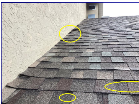
Roof covering showed signs of curling, cracking, and aging.
