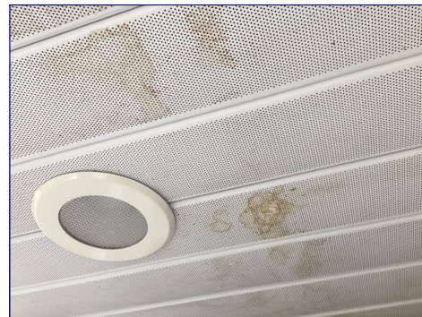
Soffit shows water penetration. This is most likely caused because of water leaking through from above. I recommend a licensed roofer evaluate the shingles and the flashing between the walls and the roof.
