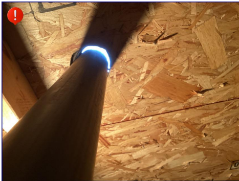
The plumbing vent stack is not properly sealed at the entry through the roof. I recommend a roofer repair this issue.
