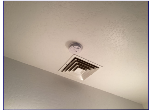
The smoke detector in the master bedroom is newer. I recommend investigating the age and making sure it is up-to-date.
