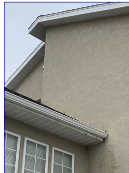
This is the exterior view where the hole in the attic sheathing is.
