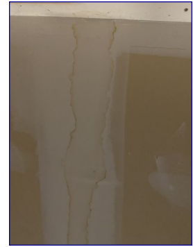
There are signs of water leaking on the garage ceiling. I recommend further investigation to determine the cause of the water staining. It could be associated with the disconnected water line and water damage in the upstairs bathroom or the non-booted vent in the attic.
