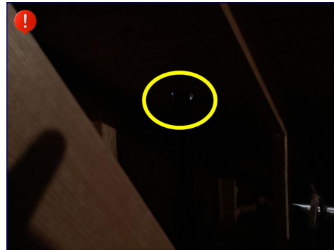
This is a picture of daylight shining through another vent stack that is not properly booted on the roof. I recommend a licensed roofer install a boot and properly flash the roof repair.
