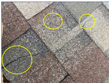
The shingles are showing signs of age through cracking. I recommend consulting with a professional roofer to determine the life expectancy of the roof.
