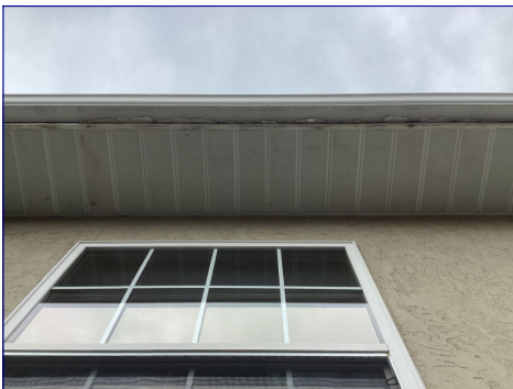
The paint is peeling on the exterior trim and soffit of the house. I recommend having these areas painted to maintain the house.
