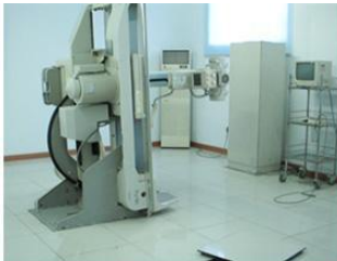
Hospital Radiology Room
