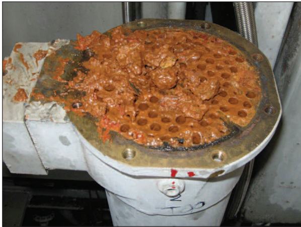
Figure 3: Unit 5 DEH cooler No. 2.
