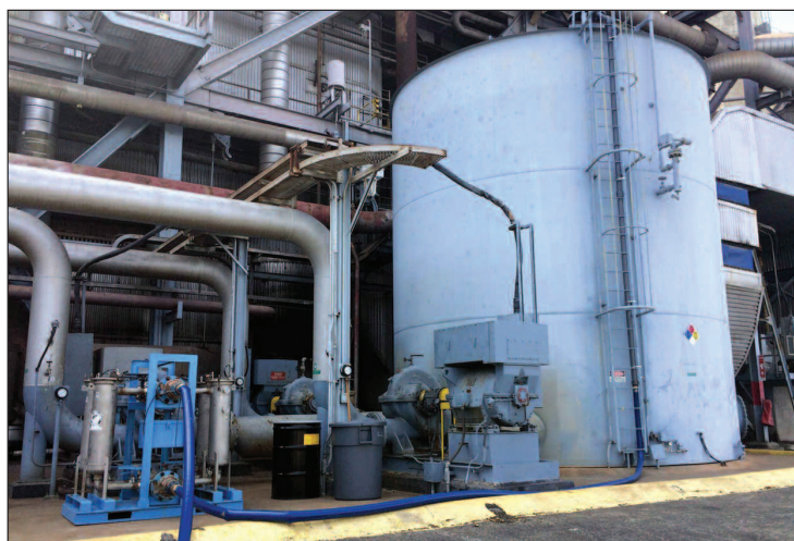
Figure 10: Filter and storage tank.
