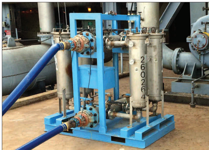
Figure 9: Skid used for side-stream filtration.
