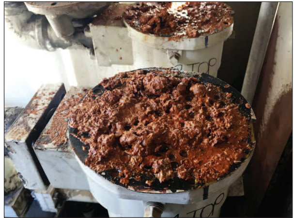
Figure 4: Unit 6 DEH coolers.
