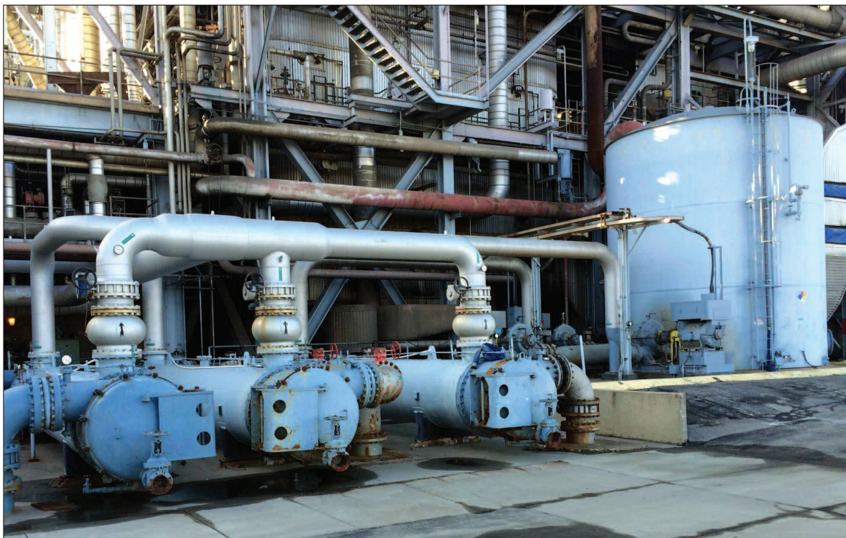
Figure 2: CCW heat exchangers and storage tank.
