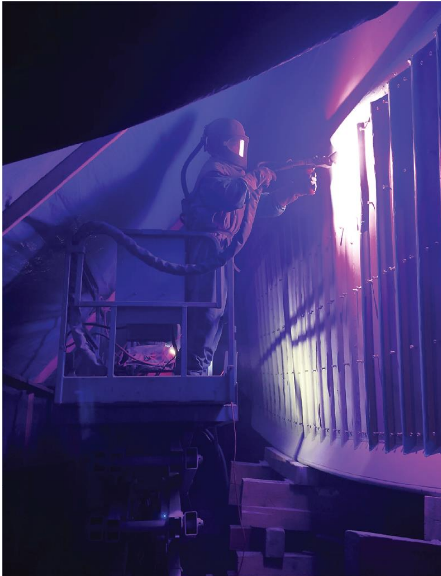
Fig. 4: Electric arc application equipment propels the molten metal onto the prepared surface with clean, dry compressed air, powered by a low-voltage, high-amperage, direct-current power source.
