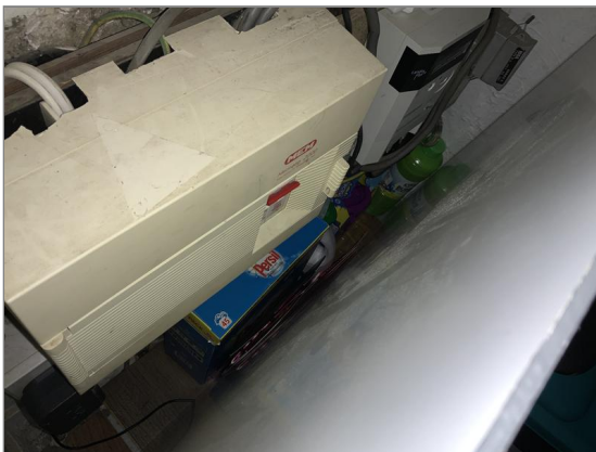
Photo - 20 Mains electricity distribution board
