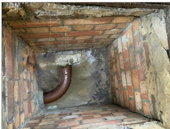
Photo - 25 Below ground drainage
