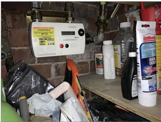
Photo - 21 Mains gas intake and meter
