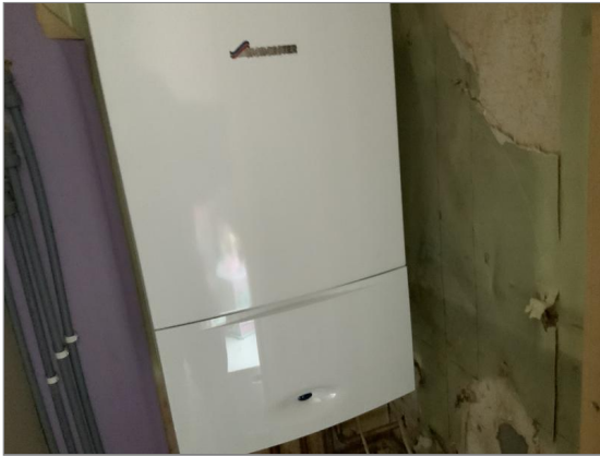
Photo - 23 Mains gas fired boiler
