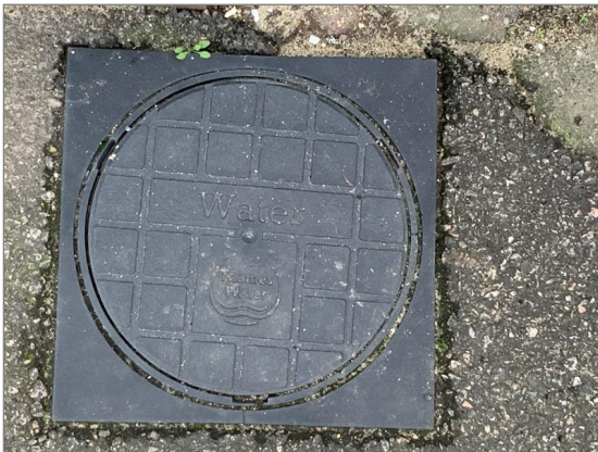
Photo - 22 Mains water intake and isolation valve
