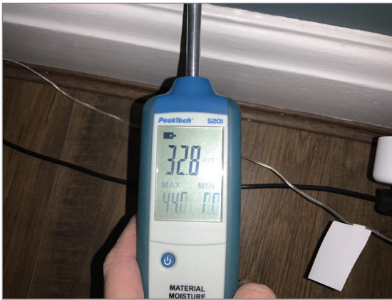
Photo - 13 Dampness within the acceptable range
