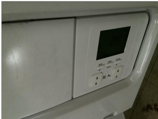
Photo - 24 Combination boiler
