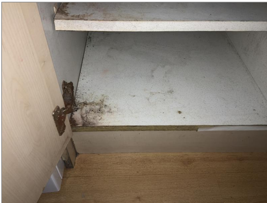
Photo - 28 Wear and tear to kitchen fittings
