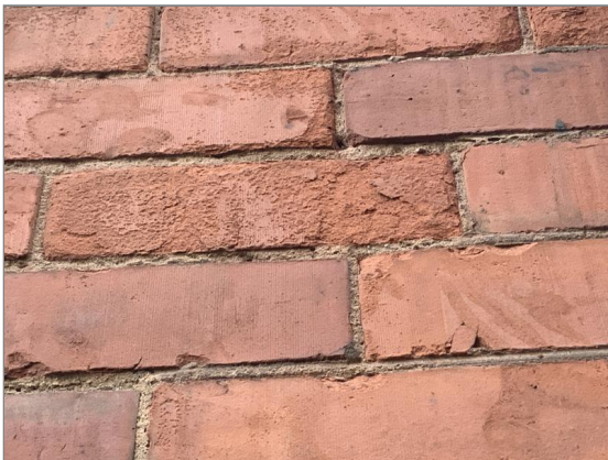
Photo - 10 Weathered and frost damaged brickwork
