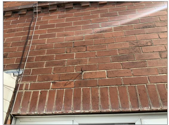
Photo - 9 Settlement fracture
