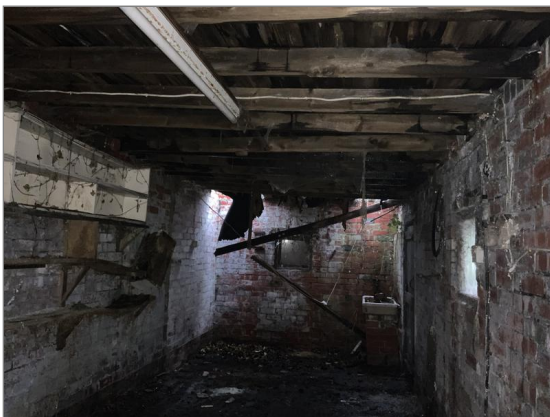
Photo - 42 Dilapidated garage
