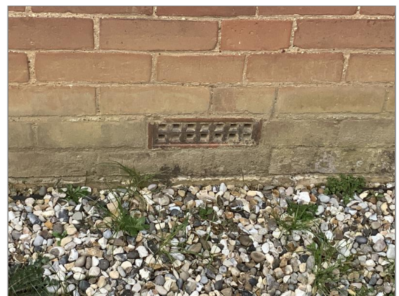
Photo - 25 Insufficient subfloor ventilation
