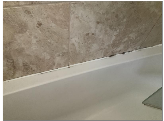
Photo - 33 Defective sealant around bath
