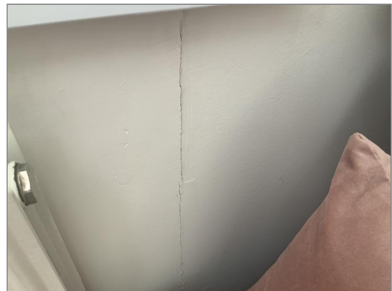
Photo - 23 Typical minor fracture to wall surface
