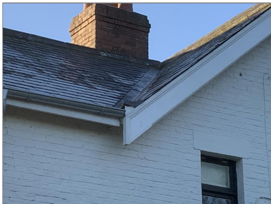
Photo - 4 Main roof coverings showing valley gutter
