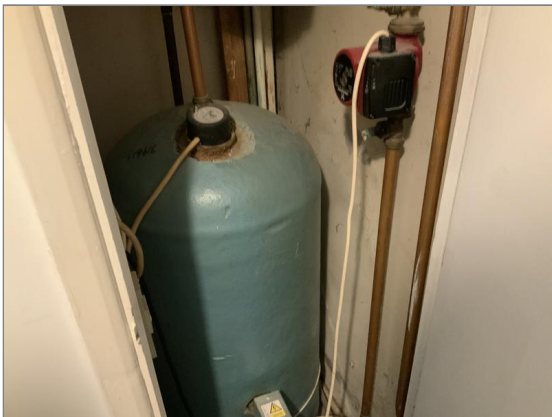
Photo - 40 Hot water cylinder
