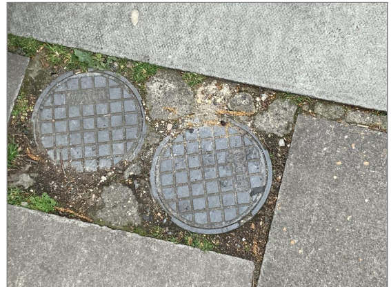
Photo - 38 Mains water intake and isolation valve
