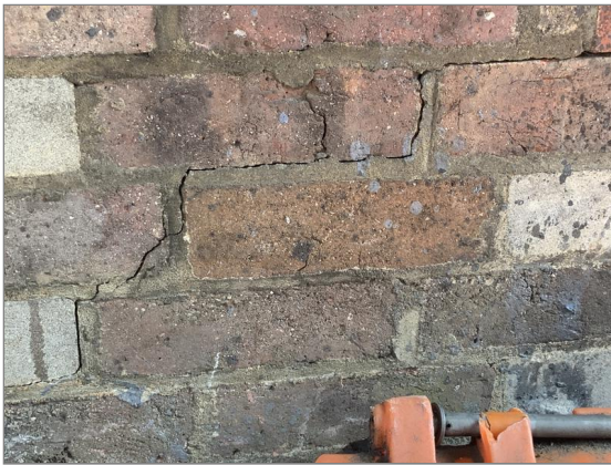
Photo - 8 Fracture to wall surface
