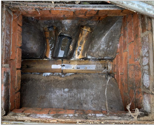
Photo - 41 Below ground drainage
