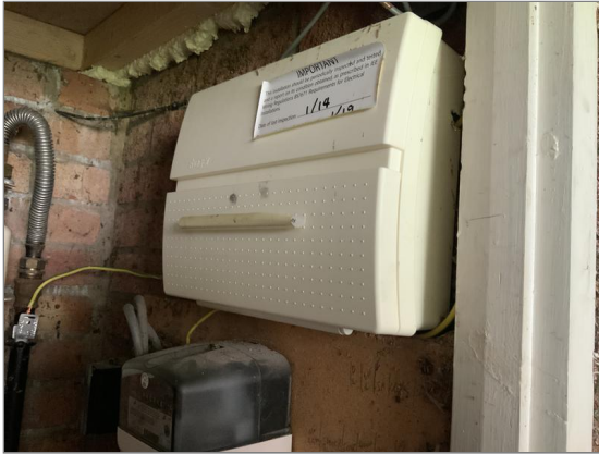
Photo - 35 Mains electricity intake and distribution board
