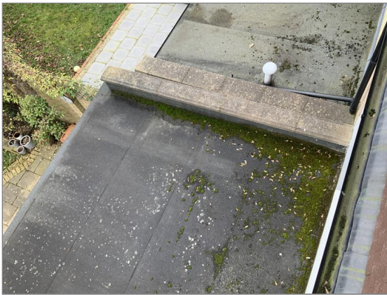
Photo - 6 Defective flat roof coverings
