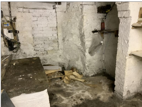
Photo - 34 Basement area - dampness and condensation
