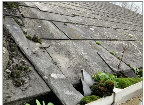
Photo - 5 Damaged slipped and missing roof tiles
