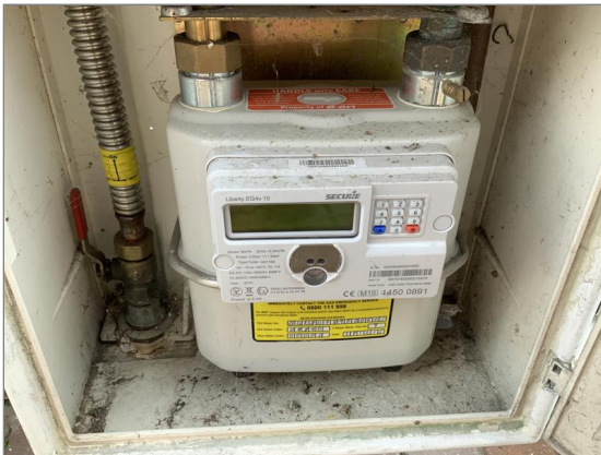
Photo - 36 Mains gas intake and meter
