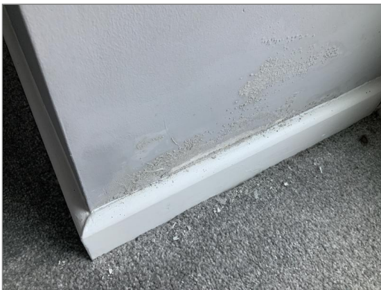
Photo - 22 Damp walls to rear
