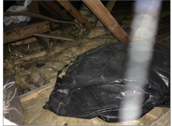
Photo - 17 Insufficient insulation
