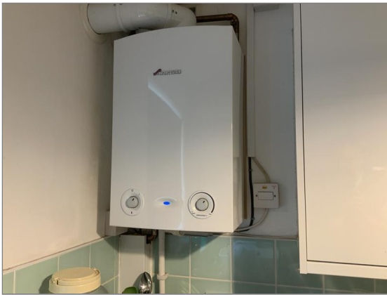
Photo - 39 Mains gas fired boiler
