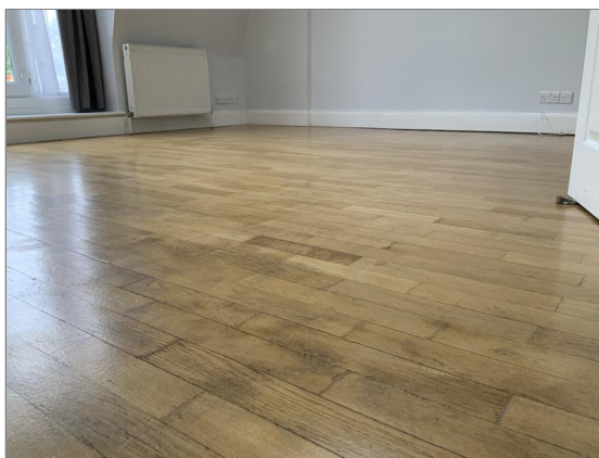
Photo - 24 Uneven floor surfaces
