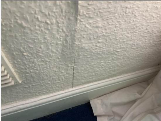
Photo - 20 Damp wall surfaces
