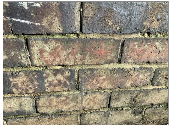
Photo - 11 Eroded mortar pointing to brickwork
